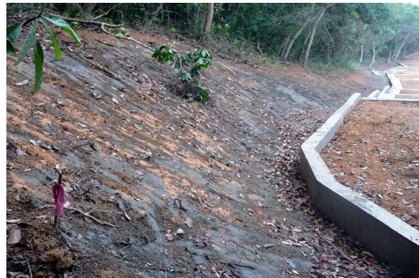
slope scuffed with cement
