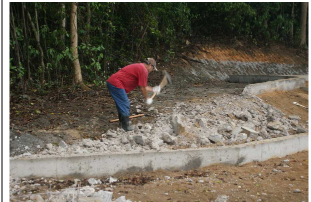
清拆霸佔官地 Clearance of Illegal March 4 2009 Demolishment of illegal occupation of Government Land
